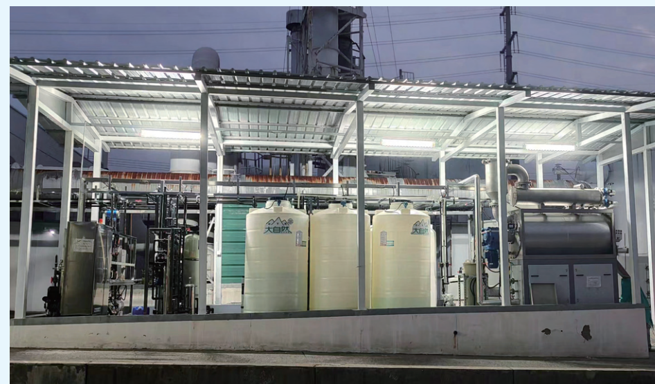
Zero water discharge treatment system
