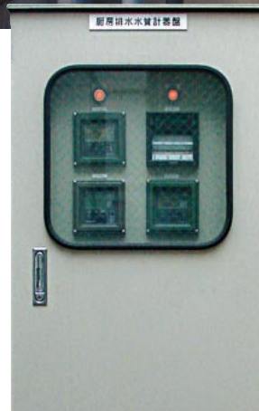
Canteen Effluent Quality Monitoring Panel (at Headquarters)
