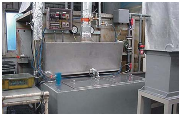
New Separation Tank (in Kofu plant)
