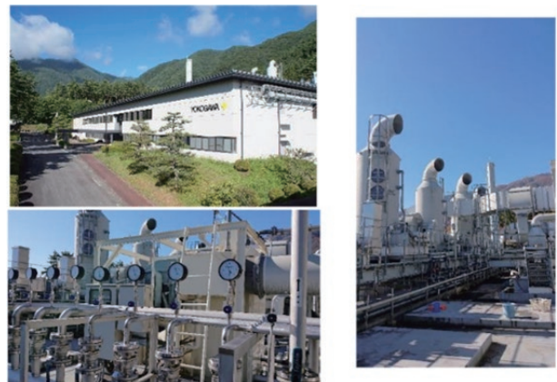
Figure 4 Building exterior and rooftop inspection area at the Yokogawa Manufacturing Komagane Plant
