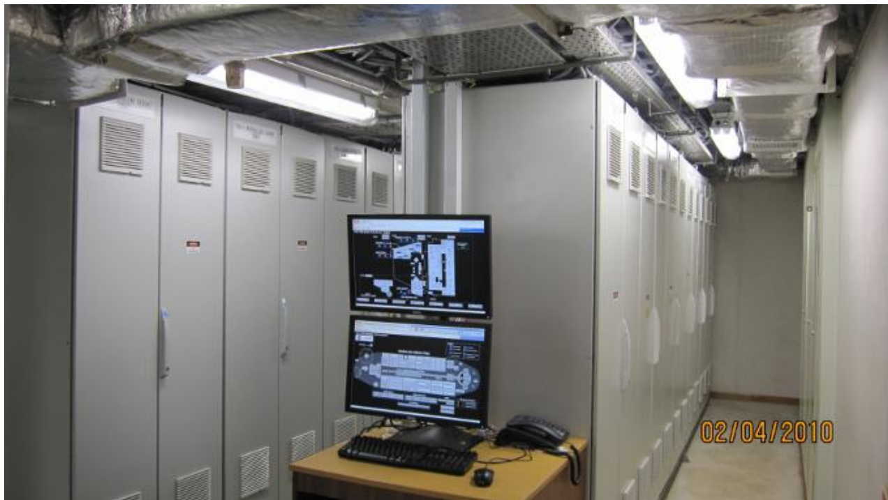
Instrument technical room
