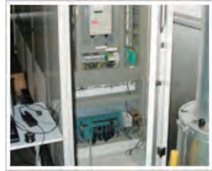
STARDOM controller installed in the site cabinet
