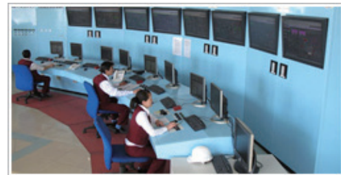
Boiler control room
