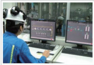
Main control room
