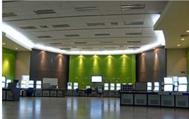
Central control room
