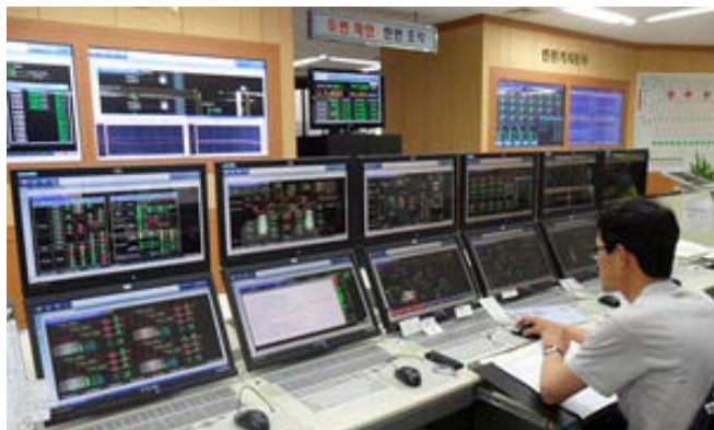
CENTUM VP operator in central control room
