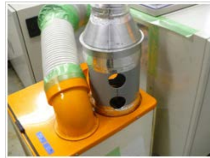
Countermeasure to exhaust heat from spot cooler
