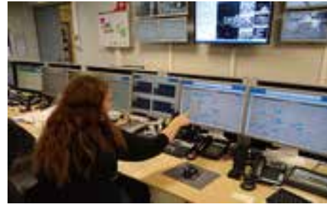
One operator per shift in the central control room
