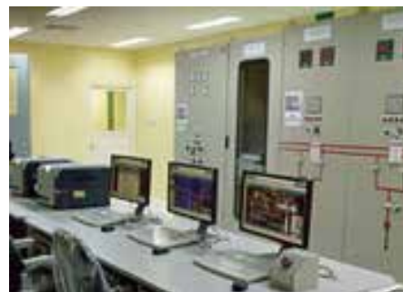
Central control room
