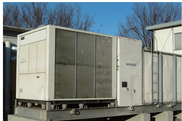
Ice-storage chiller (cooling device)
