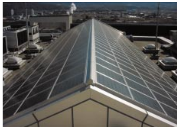
Solar-electric Power Generation System on Rooftop of Technical Center
