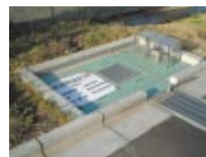
Spill-out Prevention Pit (in Kofu plant)
