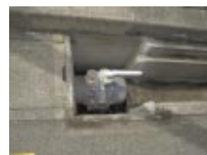
Drainage Shutoff Valve (in Nagano plant)
