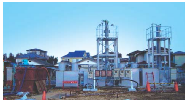
Entire View of the Pumping-up Purification Facility
