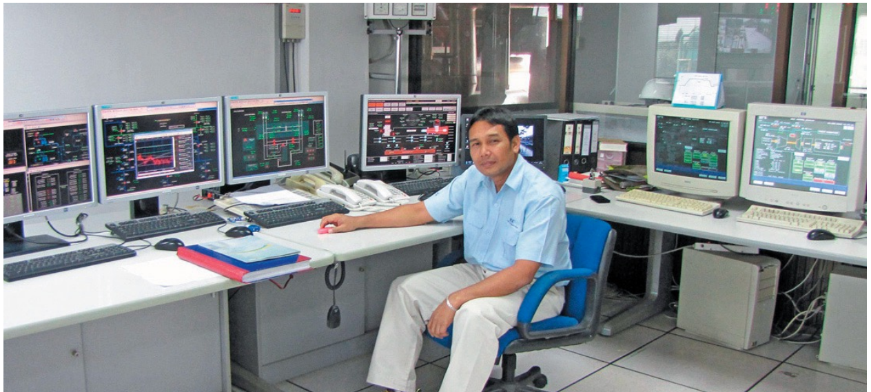
Central control room
