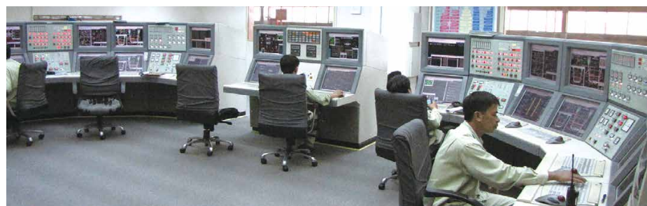
Central control room
