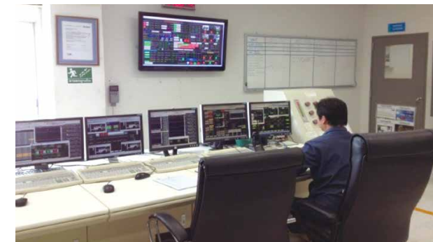
Central control room
