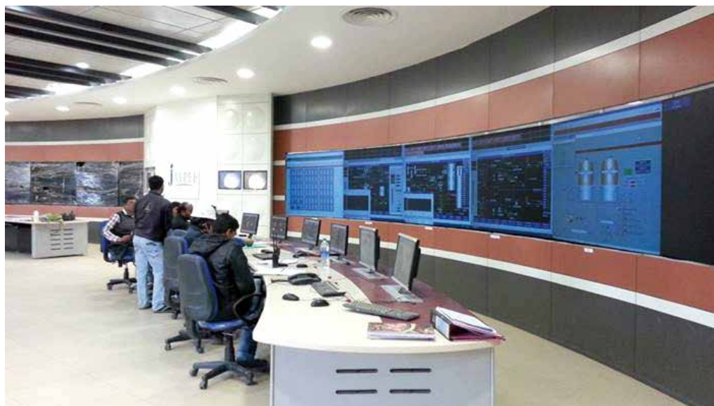
Central control room
