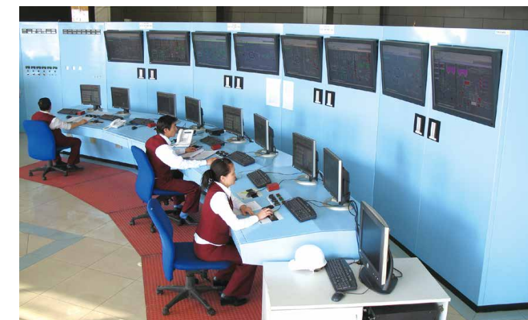
New central control room
