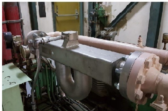
Coriolis Flowmeter in use
