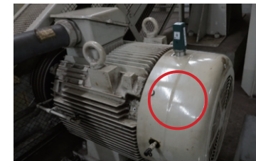
Sushi Sensor attached to an exhaust fan's motor
