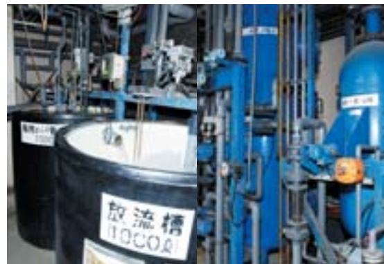
Wastewater Facility Installed in Factory
