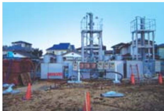
Entire Pump Purifier System
