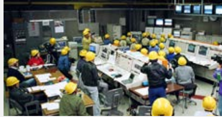
Conventional Control Room
