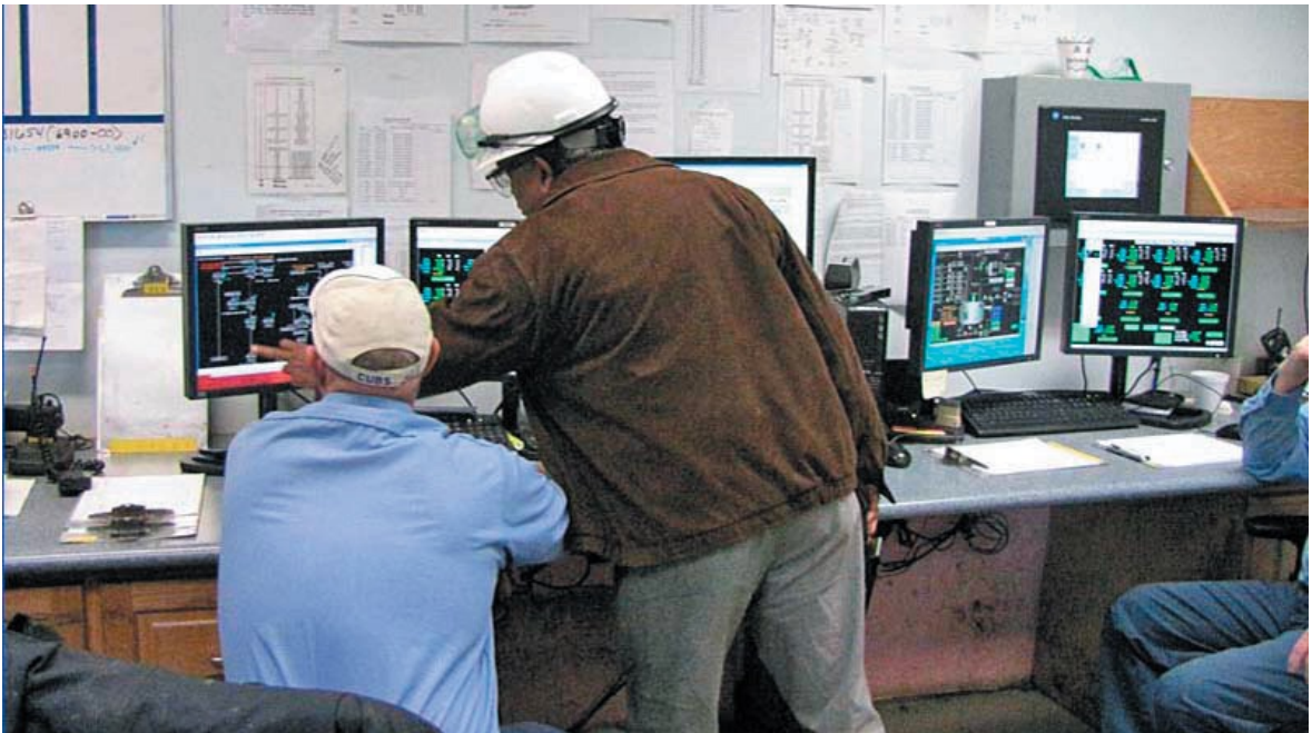
Central control room
