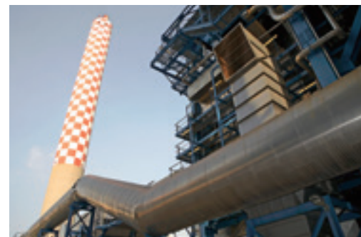
CFB boiler plant
