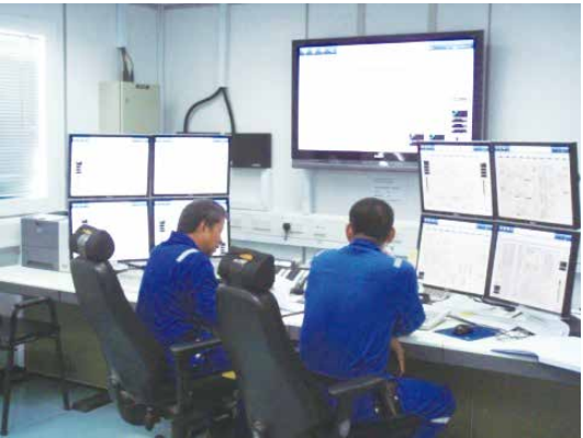
Central control room
