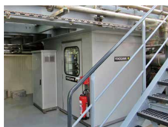
Analysis container and reserve hydrogen supply (left in attached container) at the final location
