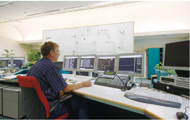
Central control room
