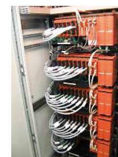
ProSafe-RS Safety system
