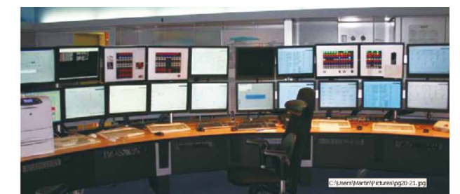
Central control room at Den Helder
