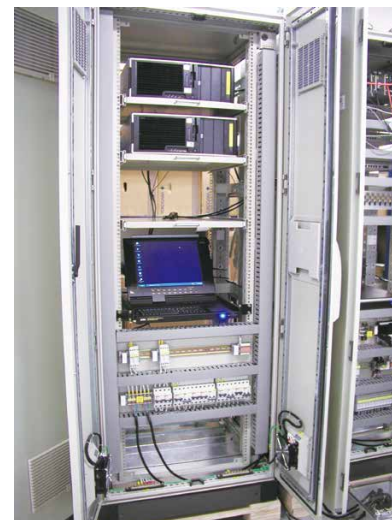
Factory Acceptance Test
