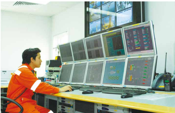
Central control room
