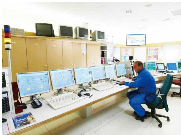
Central control room
