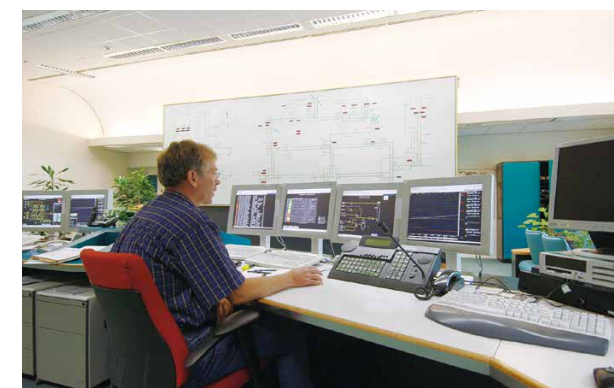
Central control room
