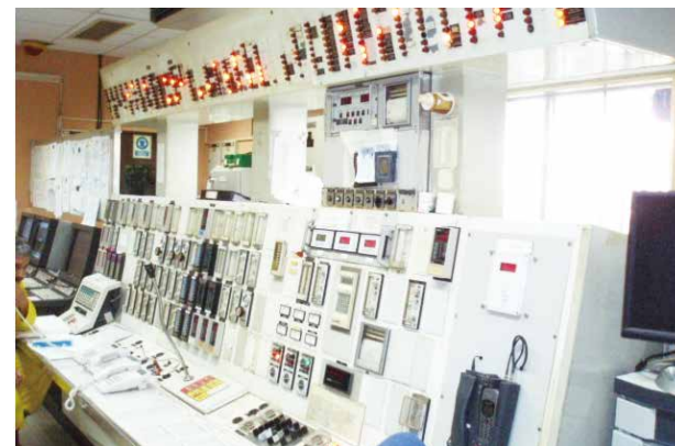
Central control room (before)
