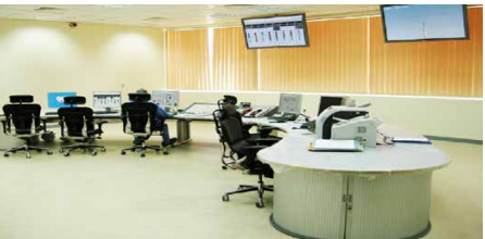
Central control room
