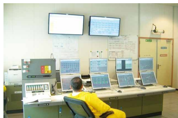
Central control room (after)
