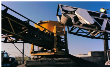
Heat Detection at belt conveyer
