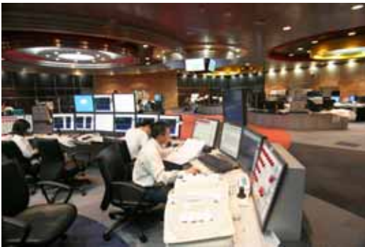
CSPC Nanhai Control Room
