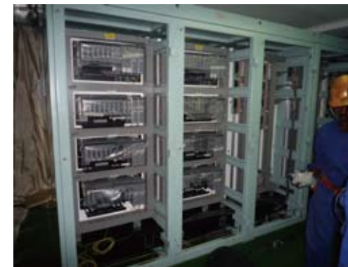
IAS Retrofit using existing cabinet
