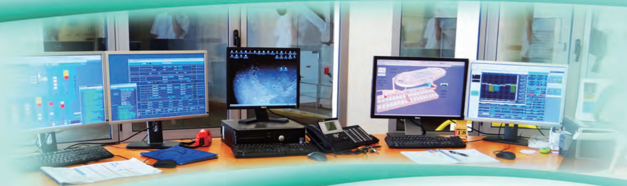
Central control room
