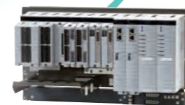
Field control station (FCS)
