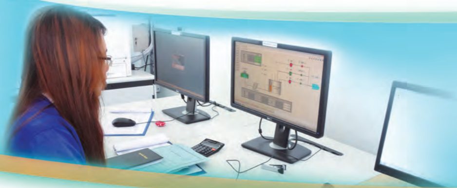
FAST/TOOLS™ SCADA system at operation room
