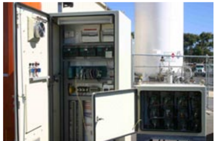
Fig.4 Automatic custody transfer system at unmanned LNG station
