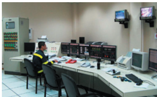
Central control room
