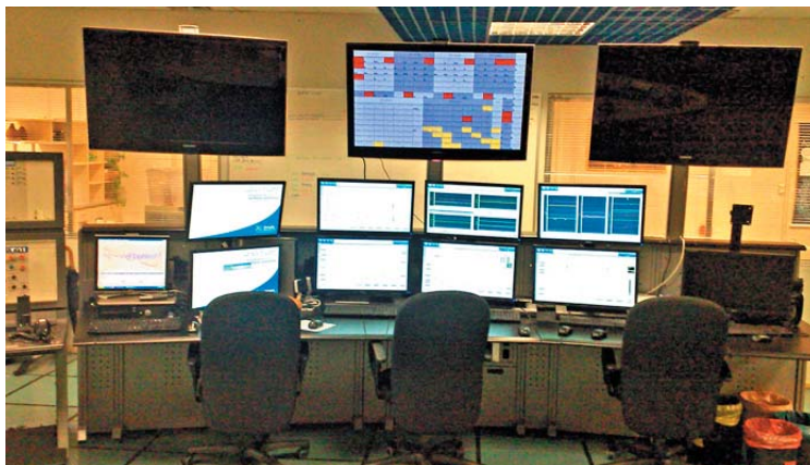
Central control room
