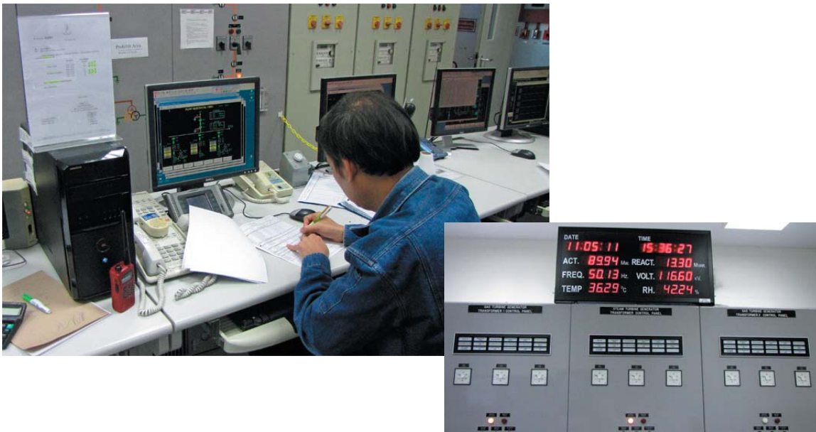
Central control room
