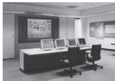
Figure 1 Example of a Modern Central Supervisory Room
