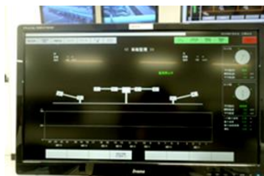
The berth monitoring system
