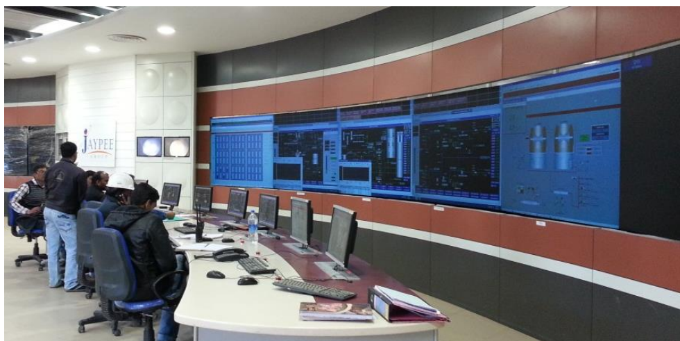
Central control room
