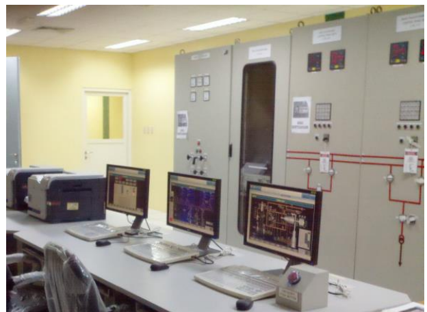
Central control room
