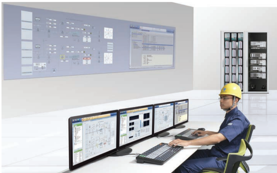
Fig.2. Yokogawa's CENTUM VP R6.01 integrated production control system
